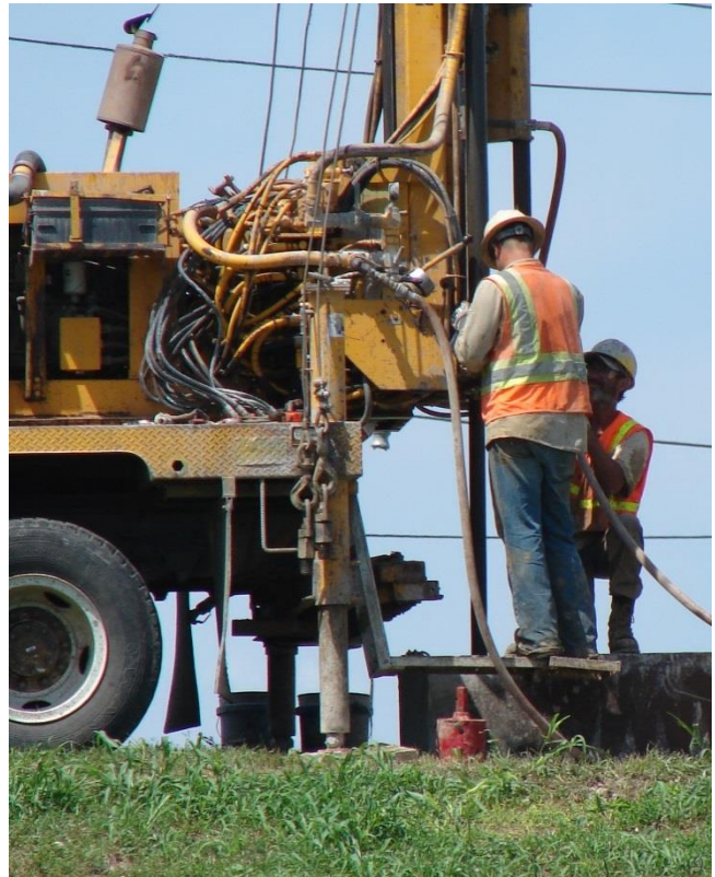
Taking soil borings for future Lamar Levee connection to the East Levee, Dallas Floodway Extension Project, Dallas.
